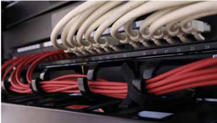
Shunting panels, zip tie/zap trap
